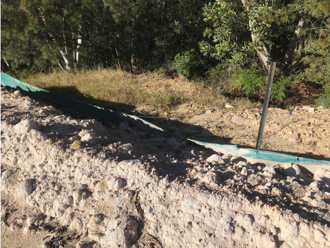
Plate 6 – Collapsed Sediment Fencing adjacent to Pit 14 Tailings Dam
