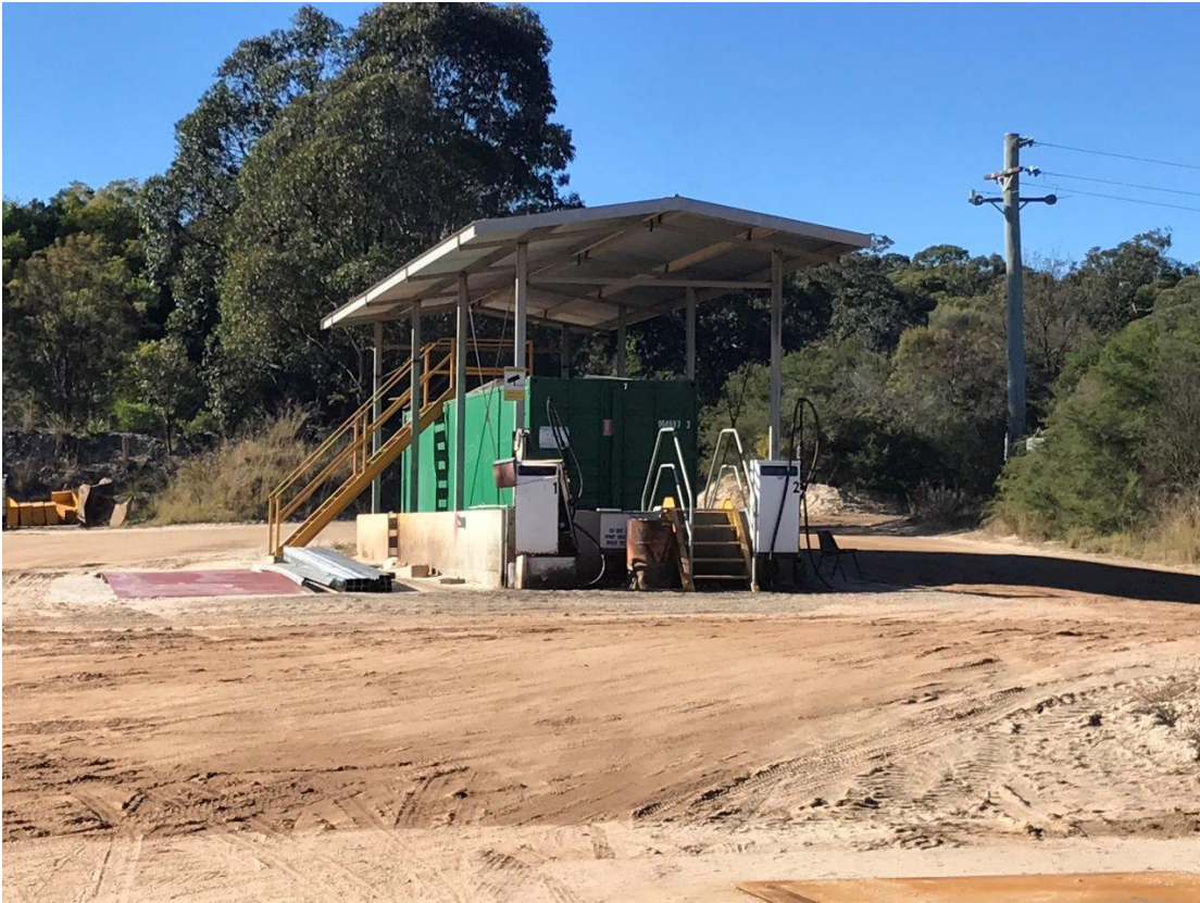
Plate 14 – Bulk Re-fuelling Bay on Lot 198
