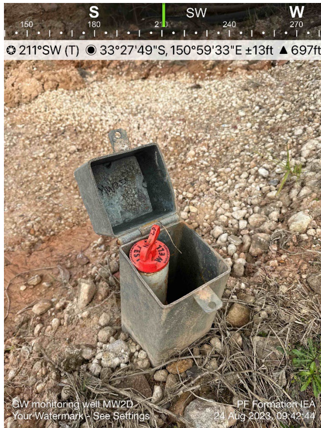
Plate 14 Groundwater Monitoring Well 20
