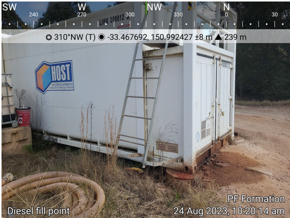
Plate 5 Diesel fill point for mobile plant and equipment
